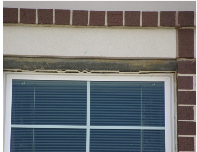
Photo 4 Sealant Joint in Need of Repair
