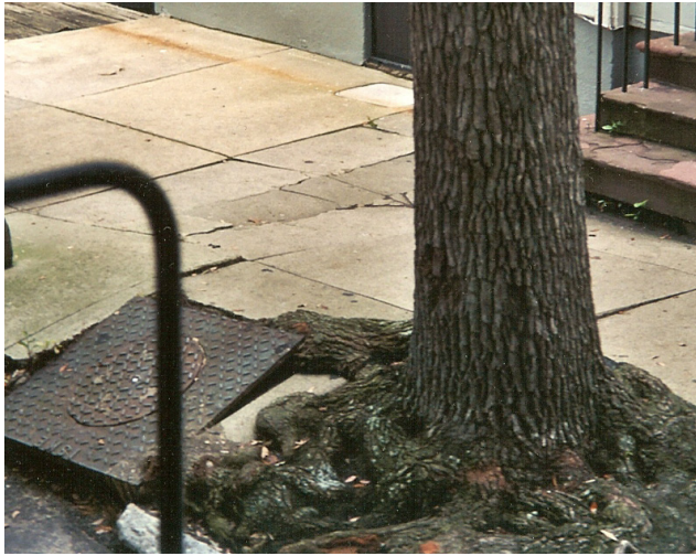
Photo 11 Upheaval of Pavements Due to Tree Roots
