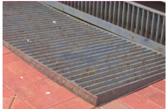
Photo 13 Abrupt Change in Level to Grate
